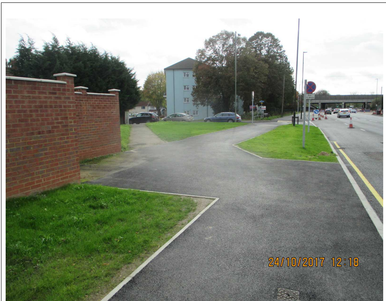
Image 4: Redesigned footway adjacent to Windsor Road at the junction with Vale Grove, looking south towards the borough boundary. Taken mid-scheme 2017
